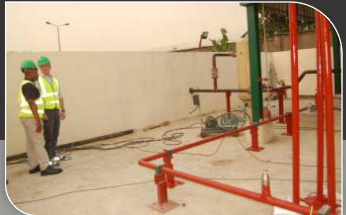
CNG plant installation 1
